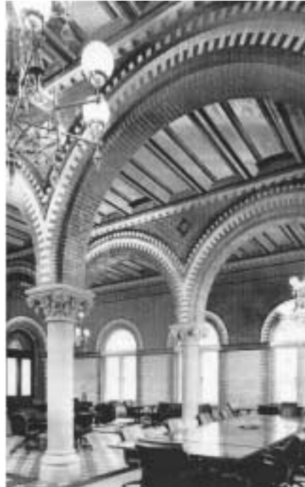
Fig. 5. Restored courtroom in the south wing. This courtroom, designed by Leopold Eidlitz, has tile floors and polychromed-brick jack-vault ceilings. The bottom flanges of the rolled-iron beams supporting the jack vaults are exposed. The reproduction chandeliers provide the principal illumination for the room, using frosted tungsten halogen lamps. The historic fixtures also serve as emergency lighting throughout most of the building; they are wired to emergency circuits that are activated by the fire- and smoke-detection system. This arrangement alleviates the need for modern emergency-lighting fixtures, which would be visually intrusive in the historic spaces. Because the detector heads for the air-sampling smoke-detection system are incorporated into the lighting fixtures, they are not visible in the room. Photograph by Lily Wang.
